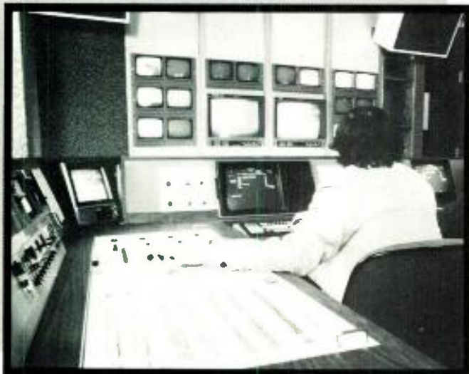
In ABC's new post-production room monitors are in wall above edit position, switching directly under operator's left hand.
